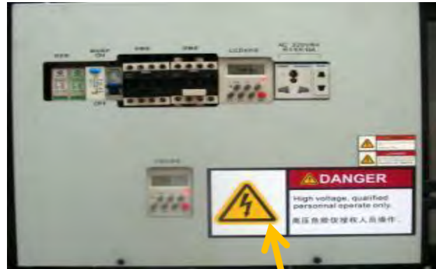
AC power control module
