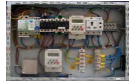
AC electrical control module
